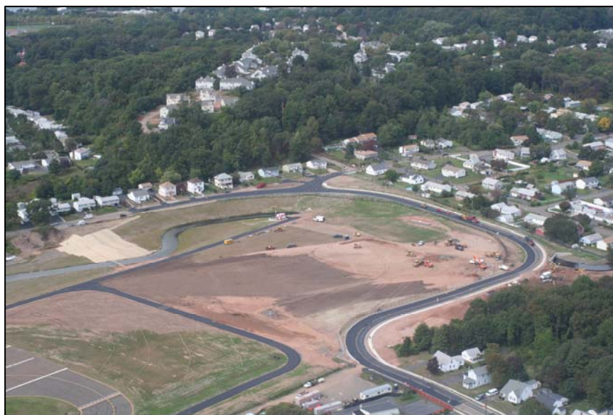
Construction of RSA North and relocation of Dodge Avenue in the summer, 2009.
