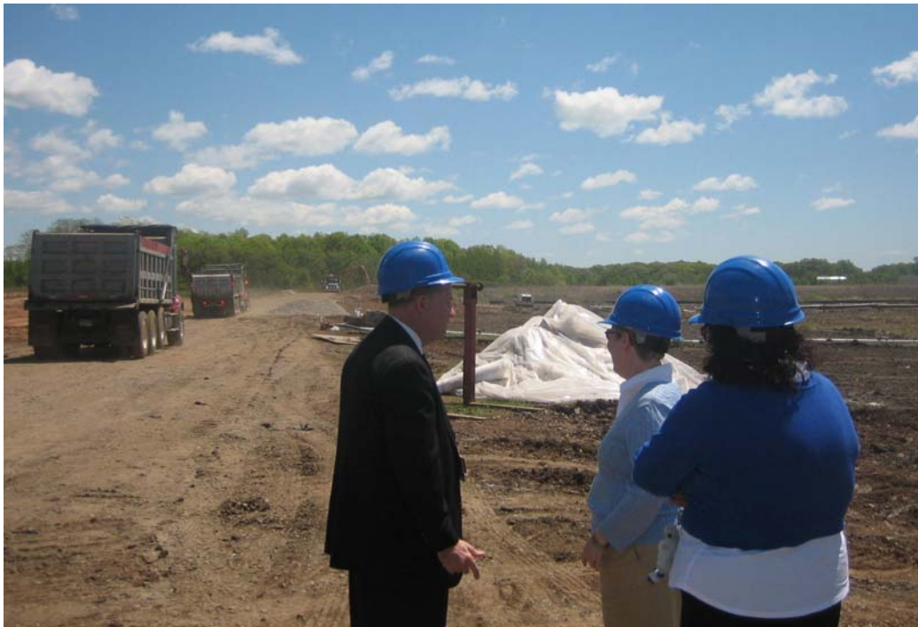
The Tweed New Haven Airport Authority successfully completed Phase I of the $24 million Runway Safety Area project. Phase 1 includes construction of the south safety area and tide gate improvements at Morris Creek. Phase 2 of the project begins in the first quarter, 2009.
