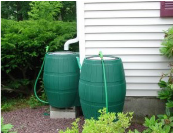
Rain barrels could be used to reduce runoff from stormwater by collecting and storing rainwater from rooftops and using it later to water plants and yards.
