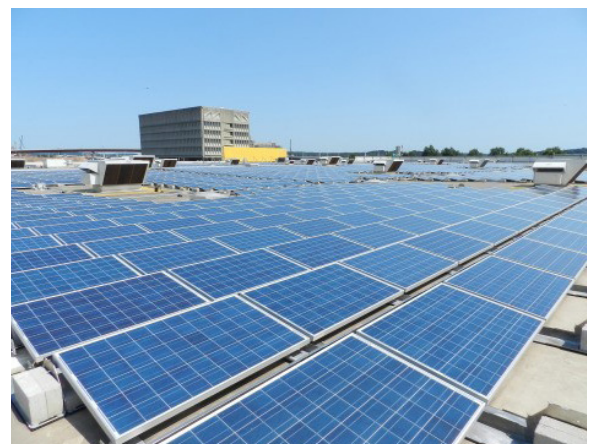
The state's largest photovoltaic array panel (3,920 panels) with a 140.8 kW system was installed on the IKEA store at Sargent Drive in 2012.
